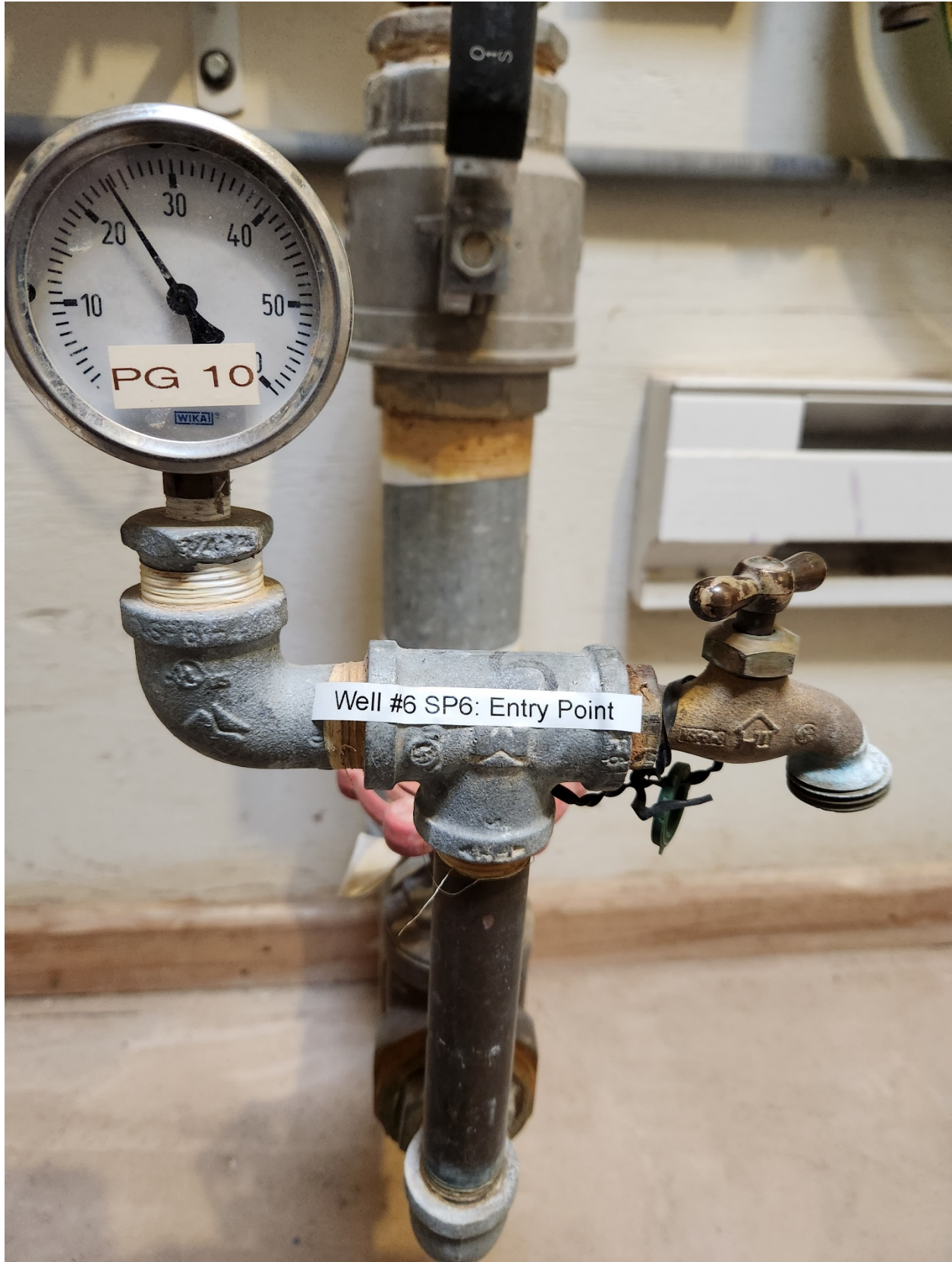
Figure 5: Well #6 Entry Point
