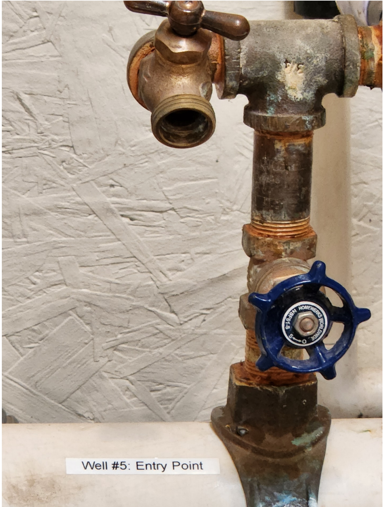
Figure 4: Well #5 Entry Point
