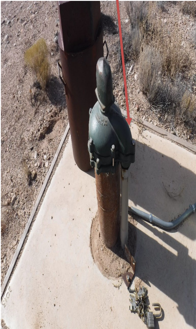
Well cap bolts loose or missing
