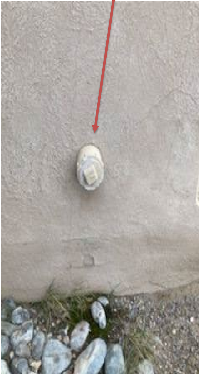
Well #5 Flush line cap leaking
