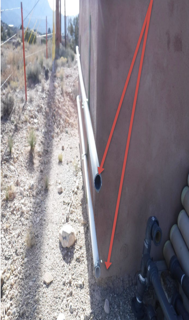
Lacking screen or needs to be replaced.
