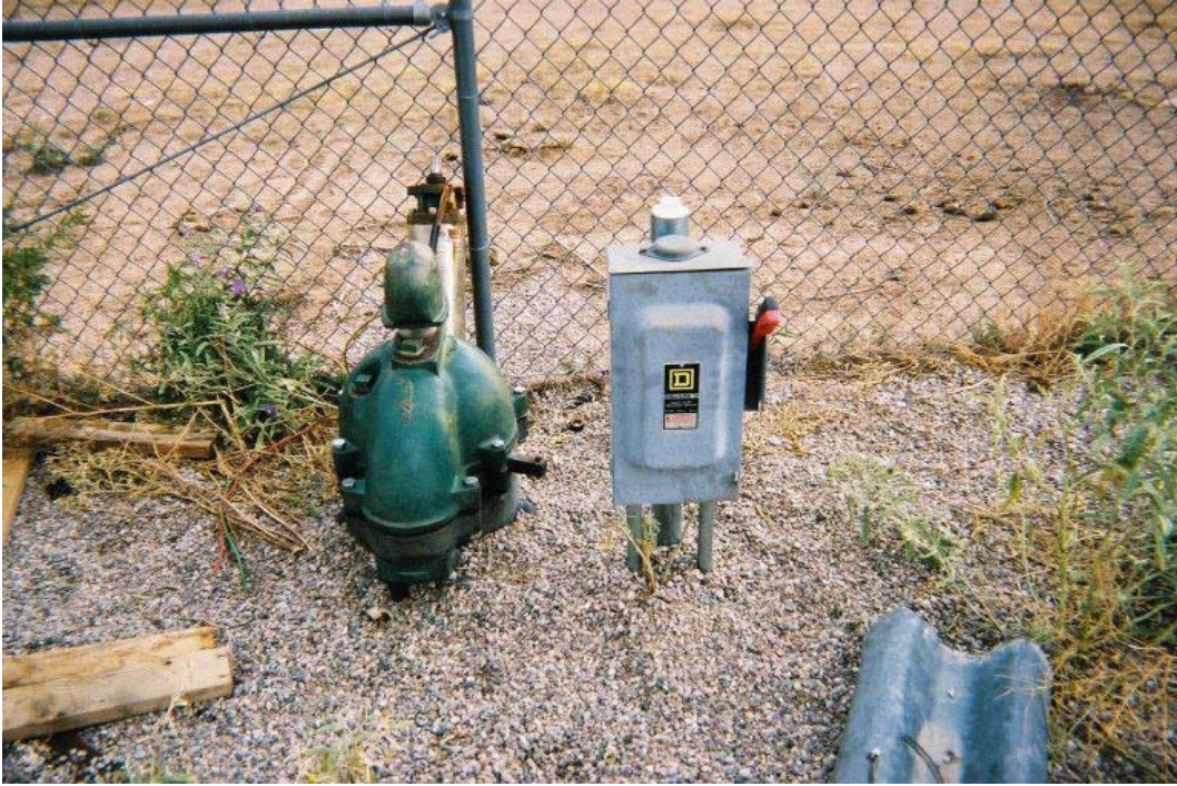
Figure 4-2. Pump Head on Buffalo Well at Nambe Pueblo, NM
