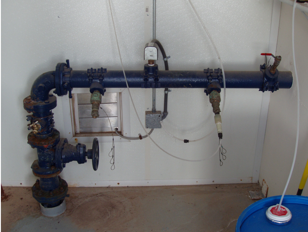
Figure 4-4. Chlorination Before Distribution at Nambe Pueblo, NM
