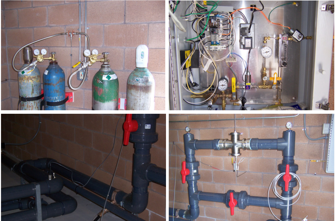
Figure 4-10. Carbon Dioxide Gas Flow Control System for pH Adjustment (Clockwise from top left: Liquid CO 2 supply assembly; Automatic pH control Panel; CO 2 Membrane Module; and Port for pH Probe)
