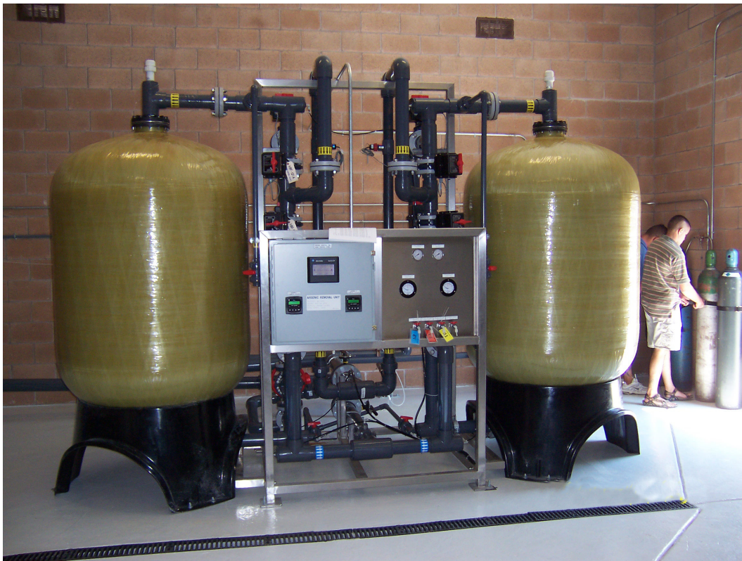
Figure 4-11. Adsorption System Valve Tree and Piping Configuration
